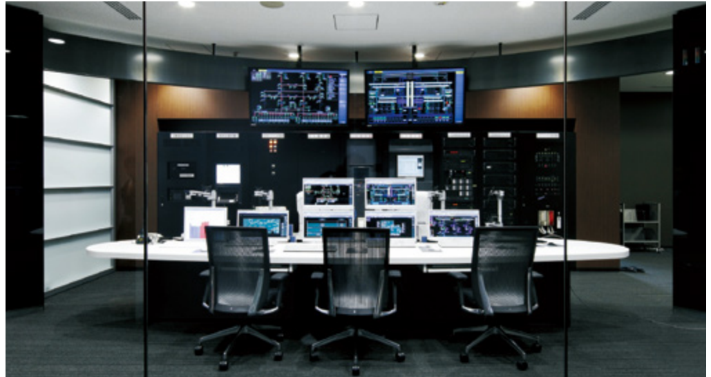
Tokyo Data Center I's operations and management center
